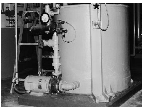
Reverse osmosis, Ósmosis invertida
